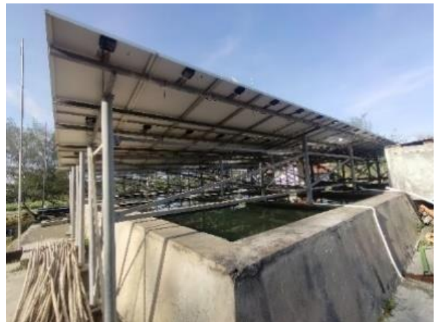
Fig.6. Pantai Baru Solar Power Plant Building
